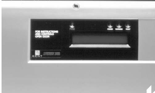
Fire Alarm Control
